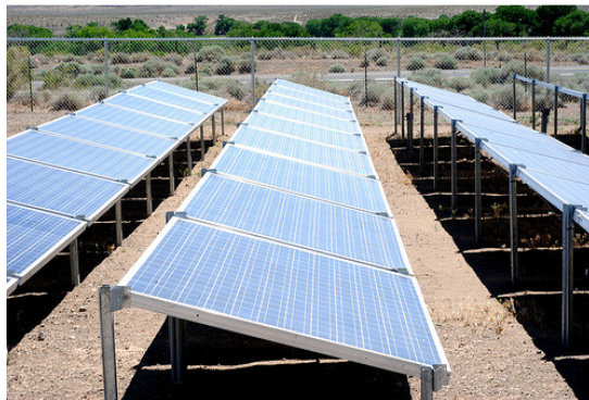
Solar Arrays at the Pyramid Lake Paiute Tribe Health Clinic. Photo Courtesy of Black Rock Solar.
