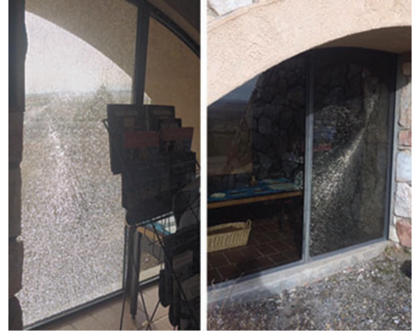
Two of the three vandalized windows that were very expensive to replace.
