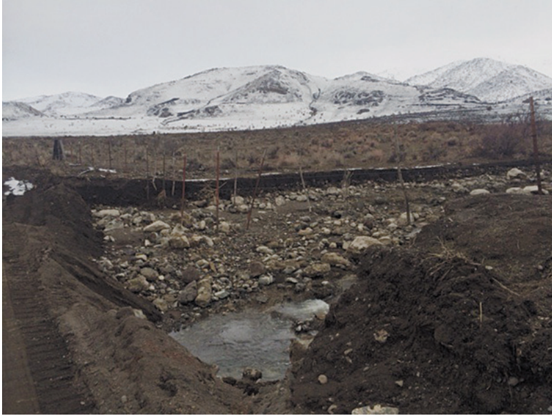
Surprise Valley Road near the Willows after the flood.
