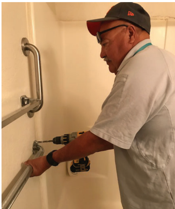
Jeff Christensen, clinic maintenance worker, installs a grab bar in an elder’s shower.
