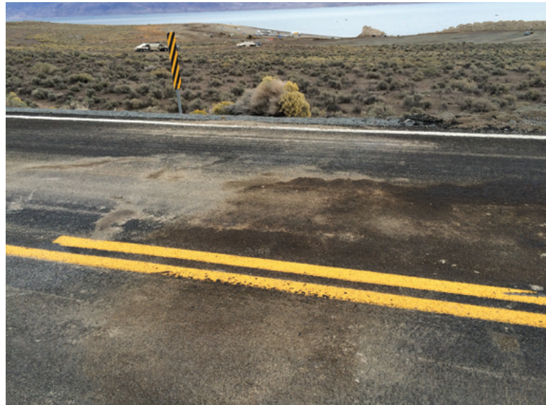
Storm water running off the roads will mobilize oil pollutants, like this oil spill near Pelican point in October 2014.
