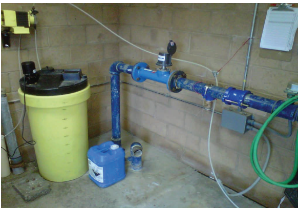
(Chemical injectors treating the water at Sutcliffe)
