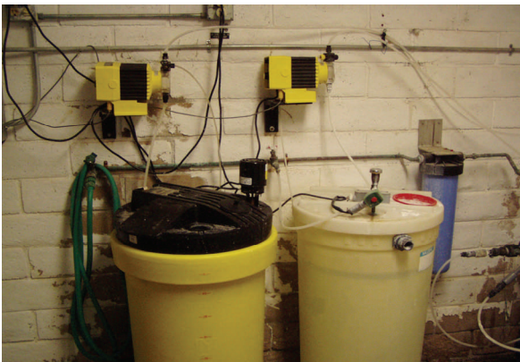
(Chemical injectors treating the water in Wadsworth)
